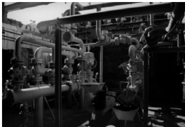
Blasting near a "Pig Launcher" on this platform required little equipment wrapping and containment due to pliant media technology's low rebound and low dust attributes.
