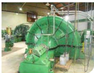
Top 3 pics: Sponge-Jet media was used to remove the previous coating and corrosion to leave a SA2.5 finish with a profile of 4mil (100 microns) for the application of Belzona materials
