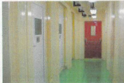
Living quarters installed on the platform
