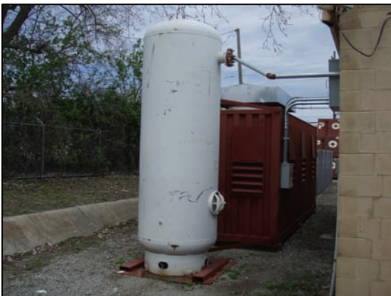
(Fig .8) 1,300 gallon (5,000 liter) receiving tank
