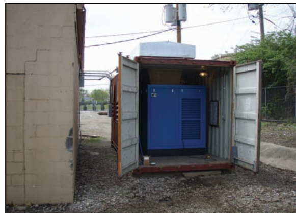
(Fig.9) 150hp, 675cfm (19.11m 3 /min) electric compressor
