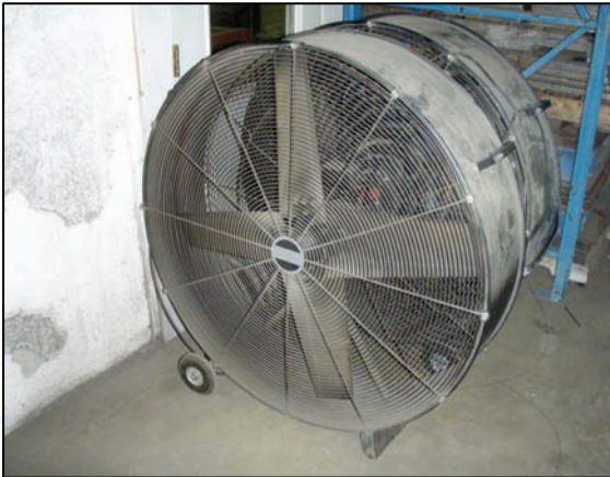
(Fig. 1) 2,400cfm fan used to reduce negative air issues
